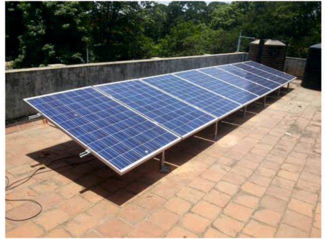
2.5 KW ROOF-TOP Installation, Thiruvallur
