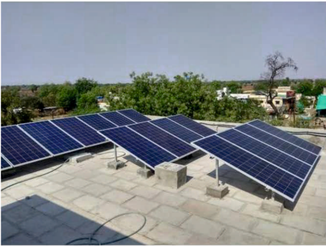
5KW ROOF-TOP Solar Installation at Chennai
